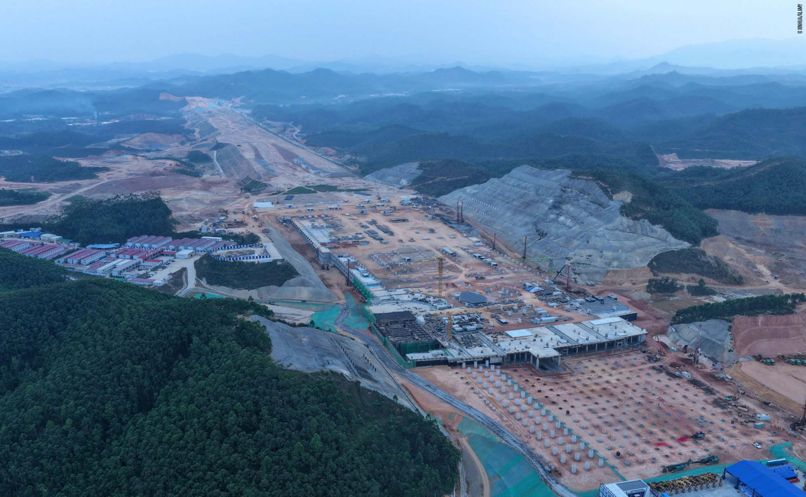
Construction work at the 41.81-billion-yuan Pearl River Delta Hub (Guangzhou New) Airport
